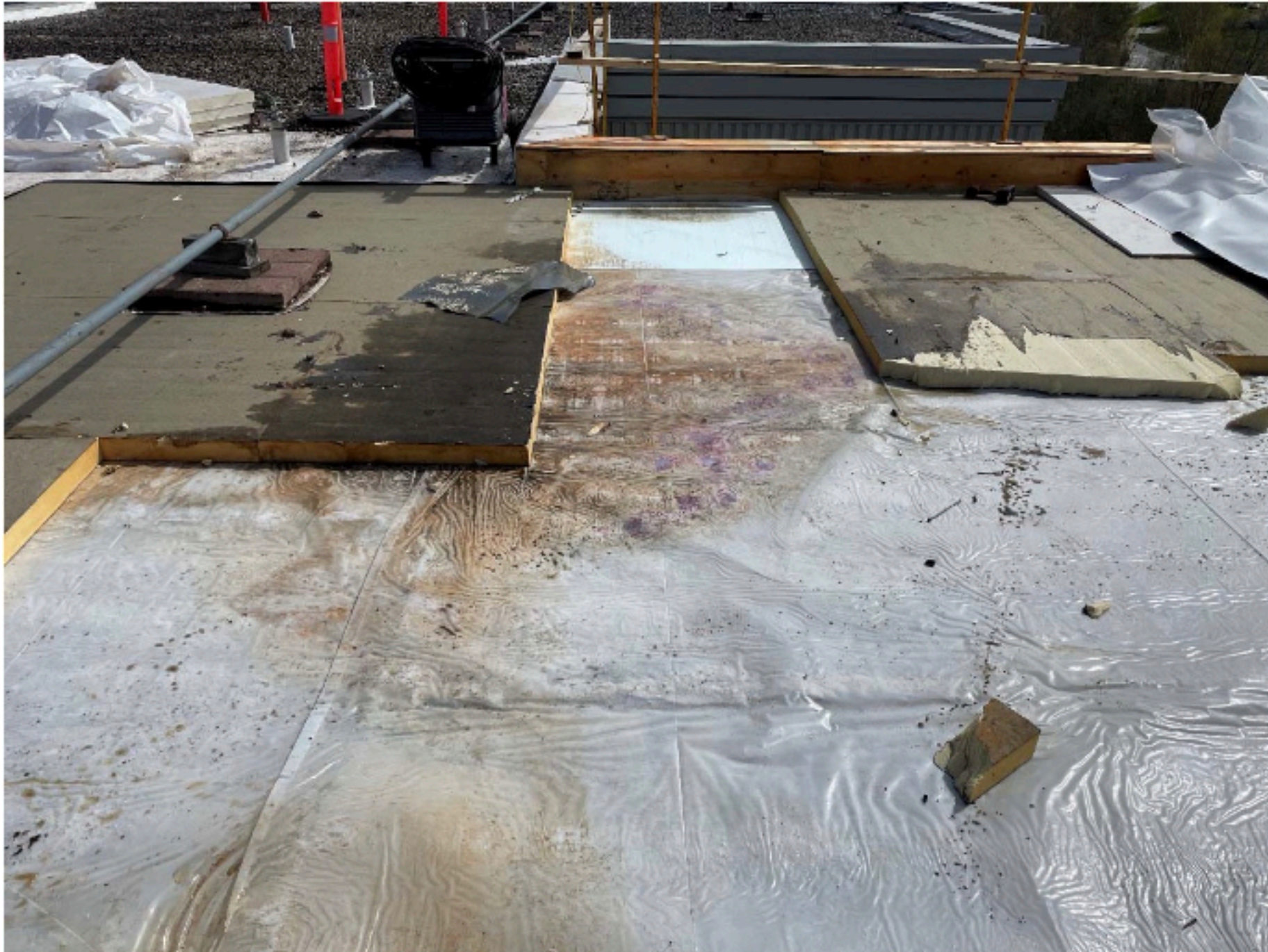
5.3 Wet Insulation, Mould and Water Under Existing Vapour Barrier
